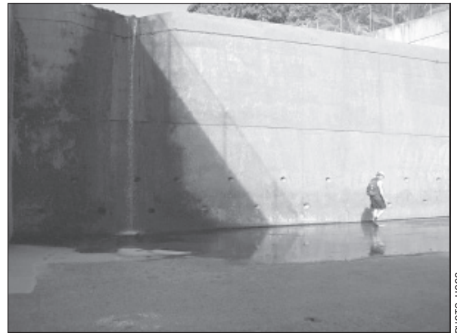
Photograph of vertical drop structure in concrete-lined channel, 'Iao Stream, Maui, Hawai'i, August 13, 2008.
